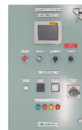
▲ Auto Control Panel
