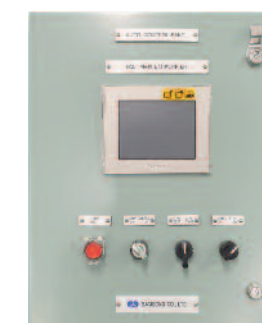
▲ Venting Control Panel
