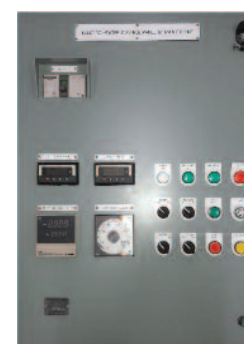
▲ Heater Control Panel
