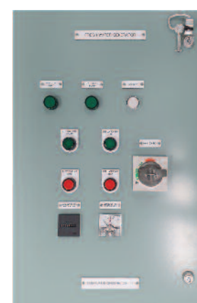
▲ Fresh Water Generator Panel
